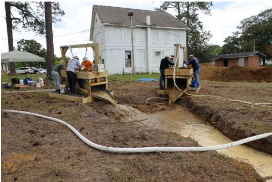
Figure 48. Water and sediment run-off into a slit trench leading to a holding pond to trap the sediment while allowing the water to run off into a natural drainage.
