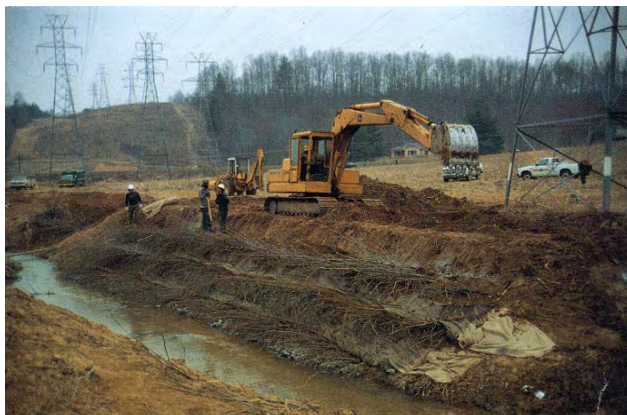
Retrofitting streambanks with willow cuttings and geotextiles can be more cost effective than riprap or concrete-lined floodways.
