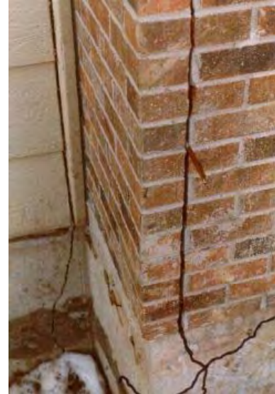
Cracks in exterior walls caused by soil expansion
