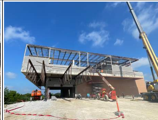
Exterior CMU on east and south side currently in progress on L2.
