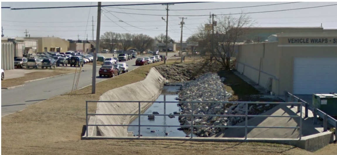
Bell Creek Tributary 11A looking downstream (south) along S. 87 th E. Ave. from the 41 st St. bridge.
