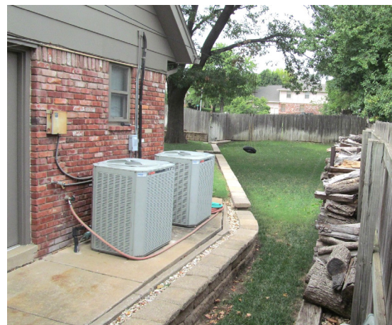
This platform and wall protect the home and air conditioning equipment from shallow flooding.
