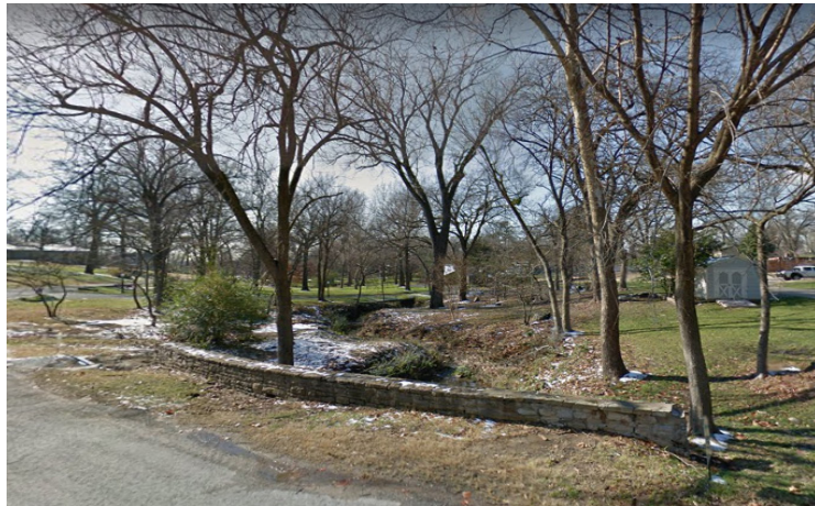
In its upper reaches Perryman Ditch Creek briefly flows in an open channel through park-like neighborhoods.
