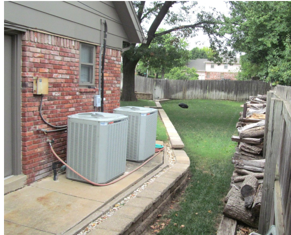
This platform and wall protect the home and air conditioning equipment from shallow flooding.
